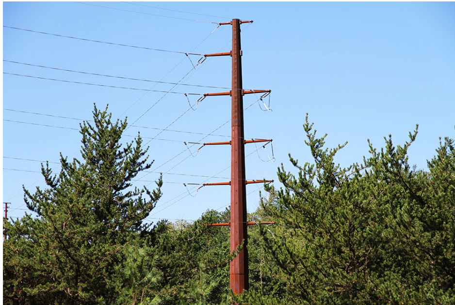
Electric transmission tower
