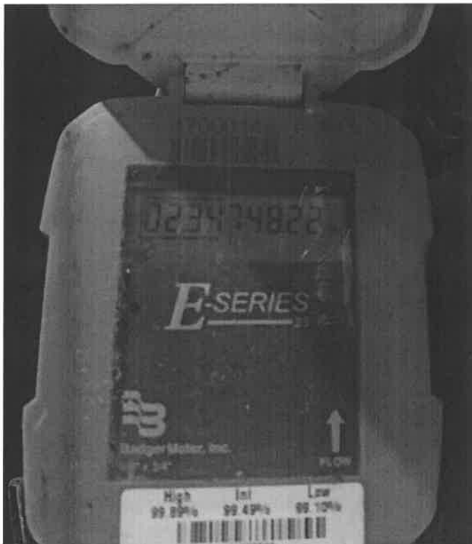
5/15/2021 at 12:04 PM 234748.22 Gallons
