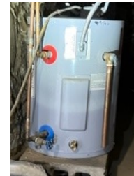
State Industries Elec Water Heater (2) 1650watt elements
