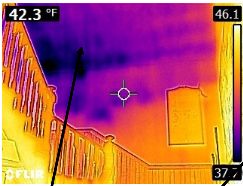
ESM 5: Blow in insulation above entrance ceiling (Access not known, possibly from ceiling hatch on northwest corner.
