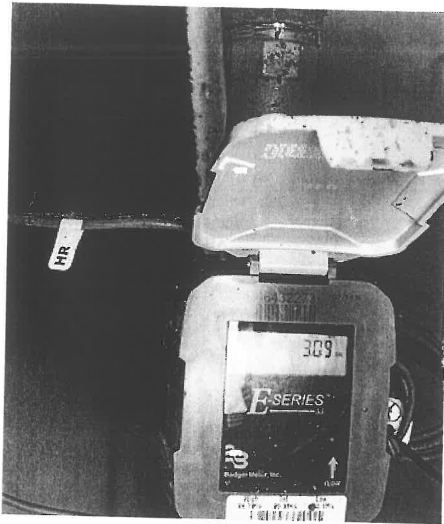
Photo of the water meter when the water is shut off in all eight trailer homes.
