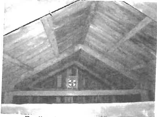
Purlins instead of ridge pole
