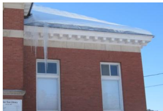
Ice damming along the eaves of the Library. Ice damming is caused by lack of proper air sealing and an inadequate level of insulation.
