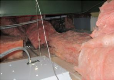
The batt insulation above the first floor of the Town Hall was poorly installed.
