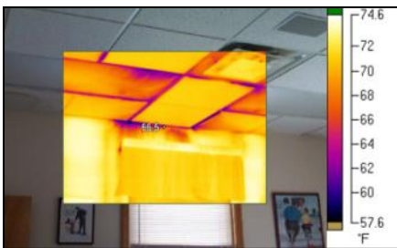
Infrared image of cold air moving from the attic space to the conditioned space at the Police Station.
