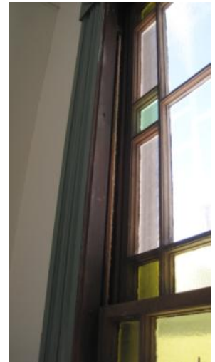
An old wood framed single pane window in Grange Hall with rope pulley. Several buildings had poor performing windows.
